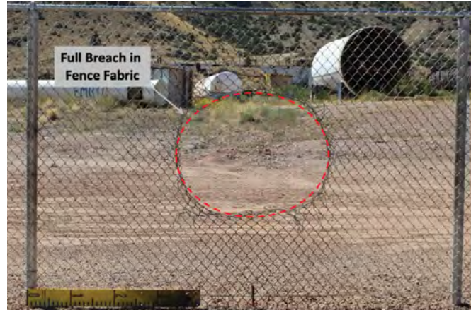
Figure 6. Explosive damage to fence.
