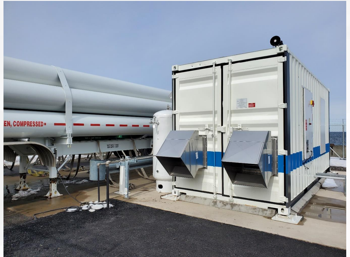
Electrolyzer and cooling unit to left Compressor below
