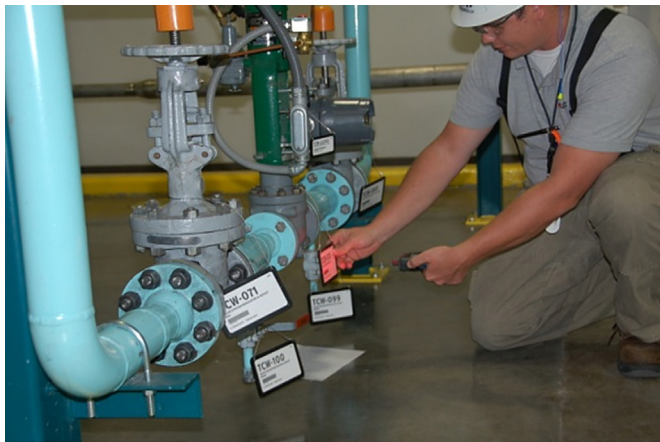
Nuclear equipment operator scanning equipment tag during Catawba demonstration.
