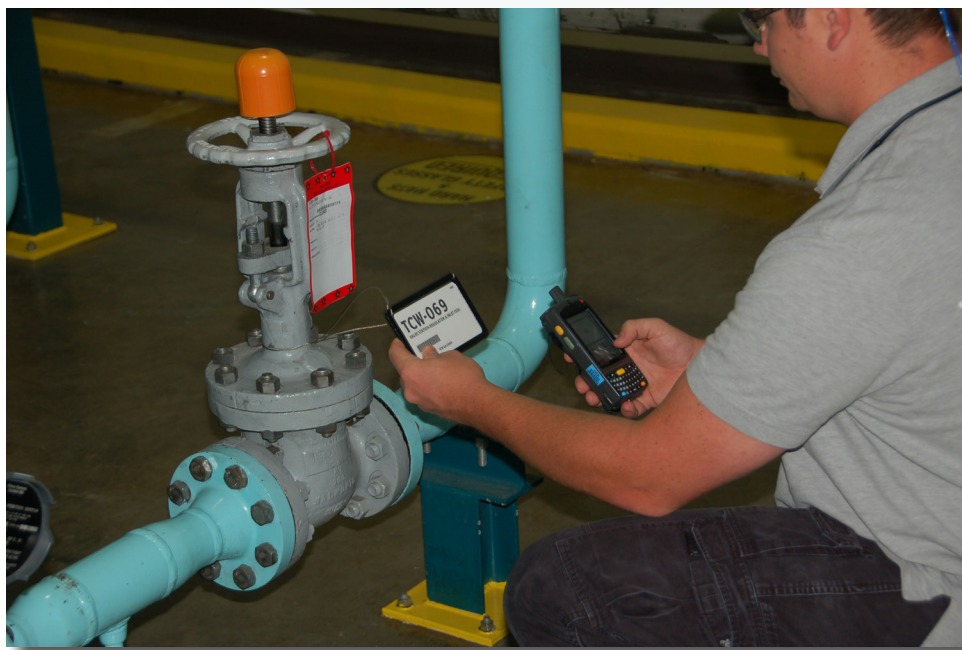
Figure 6. A Catawba Nuclear Station maintenance technician using wireless mobile worker technology to conduct valve maintenance.
